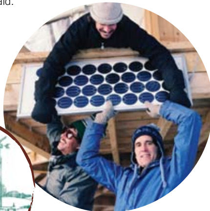
Jim Welch getting his hands dirty with a PV installation back in the day.
