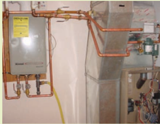
Integrated forced air space heat and domestic hot water system.
