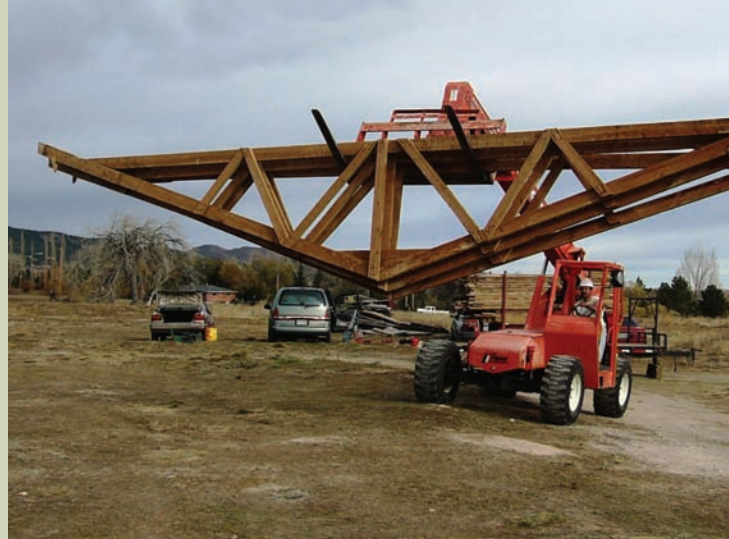
Roof joists are removed from a building to be transferred to ReSource in Boulder.
