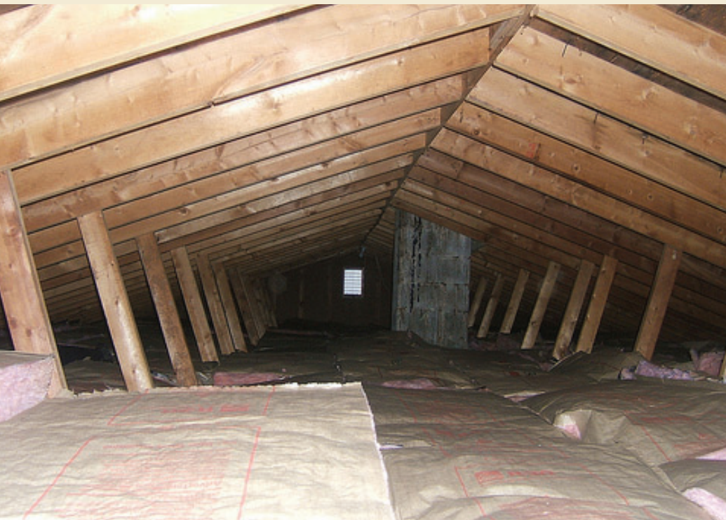
Inadequate insulation in the attic is a good indicator that your entire home is under-insulated.
