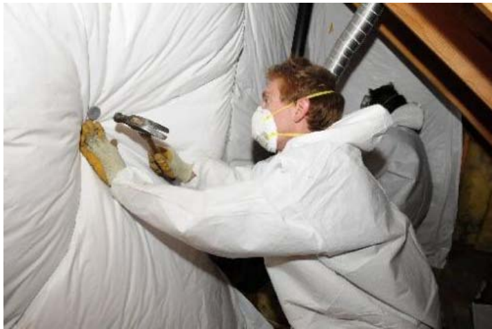
Kyle Wille, at left, and Hunter Silva work together to apply insulation to the wall of a Boulder home earlier this month. Landlords will have to make energy-efficiency upgrades to their Boulder properties -- such as replacing old furnaces, adding insulation and installing new appliances -- if a proposed set of rules is passed by the City Council next year. ( JEREMY PAPASSO )
