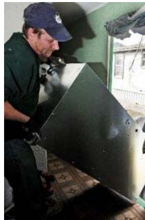
Ed Anderson of Longs Peak Energy Conservation lifts a new furnace into a mobile home last year in Boulder. Landlords will have to make energy-efficiency upgrades to their Boulder properties -- such as replacing old furnaces, adding insulation and installing new appliances -- if a proposed set of rules is passed by the City Council next year. ( CORA KEMP )
